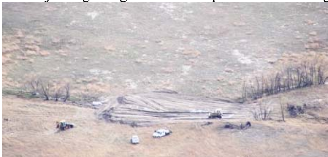
One of two structures being installed on Gracie Creek Ranch (Price's property).
