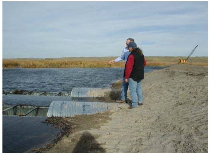
Figure 1 Twin-tube water control structure on Wolfenden.
